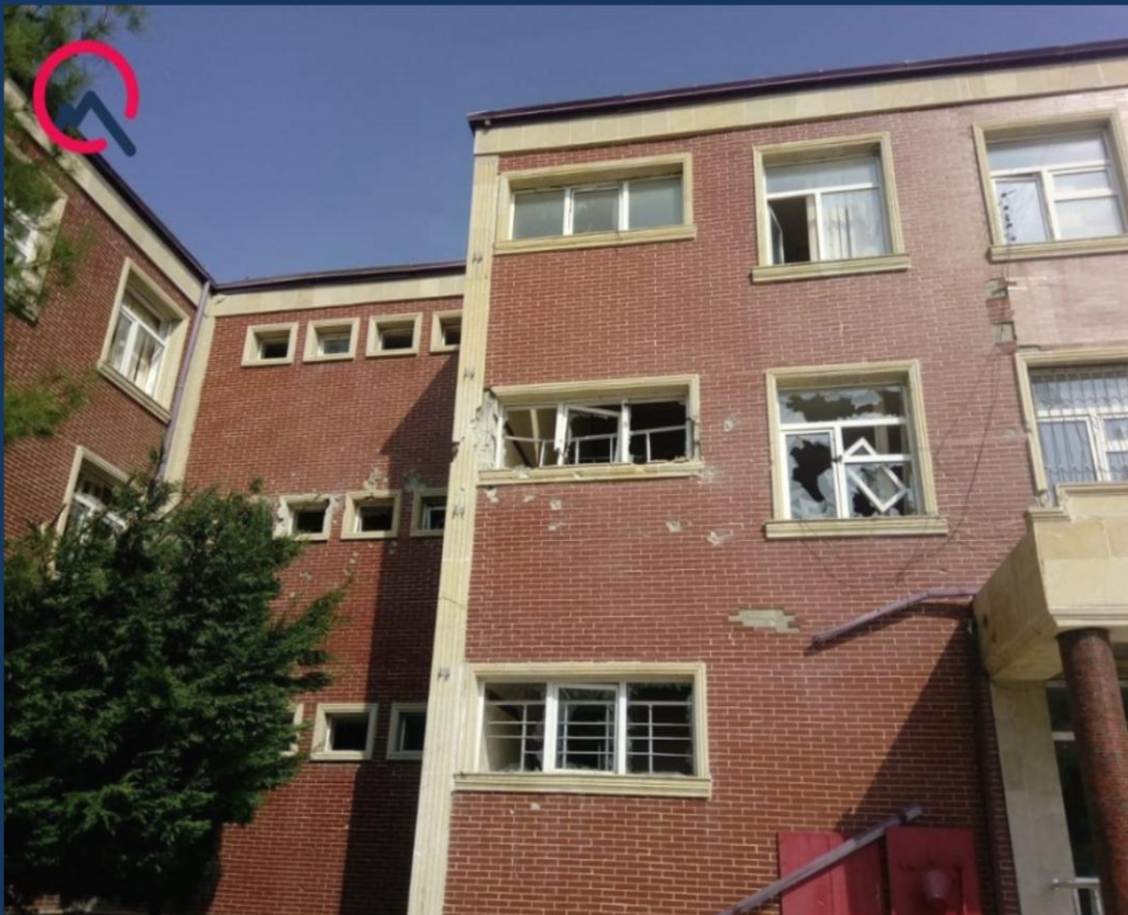
Damaged secondary school No. 1 in Tartar
